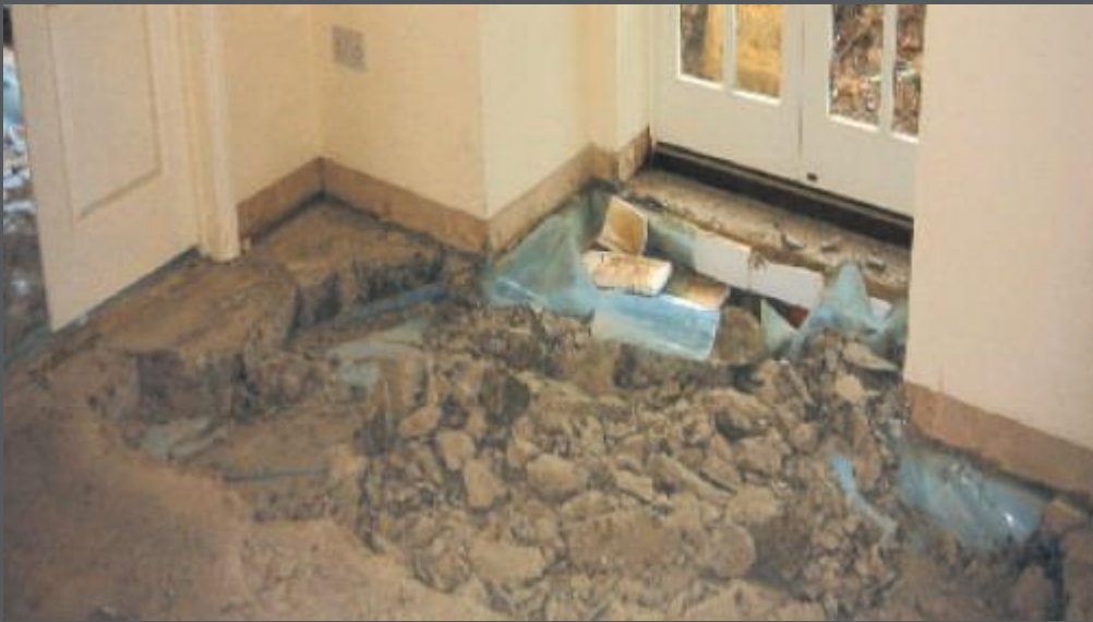
An example of a house being cleaned up following a leak of oil.
