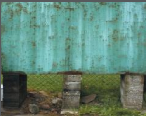
An example of a corroded tank with left hand side support stained with oil & ground soaked with oil.
