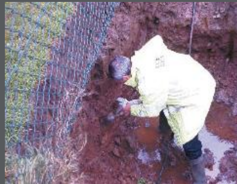
Clean up of ground after leaking tank removed, showing drinking water pipe through ground.
